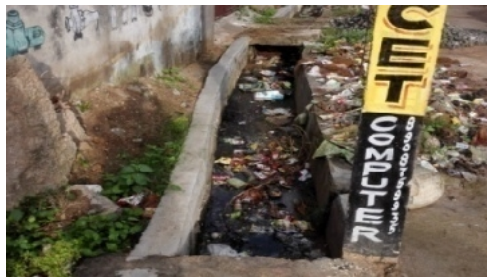
View of a choked drain
